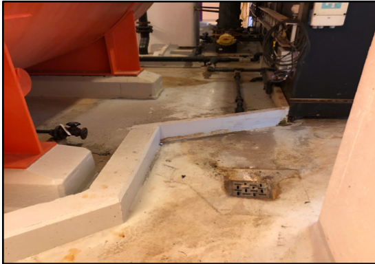
Before: damaged concrete.
