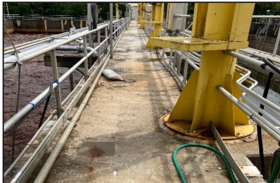
Existing coating was failing, causing the concrete to deteriorate.
