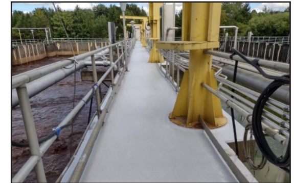
Concrete protected with two coats of ARC CS2 with a non-slip finish.
