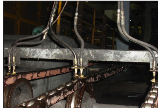
Conveyor transport chains.
