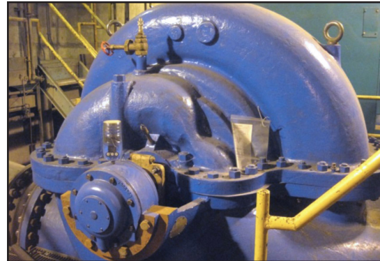
Chesterton Lubri-Cup™ EM solution installed with Chesterton 615 HTG.
