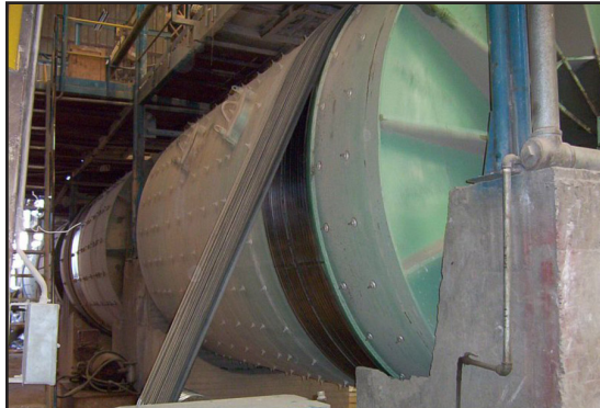
Rotary ball mill driven by 18 V-belts, which were slipping.
