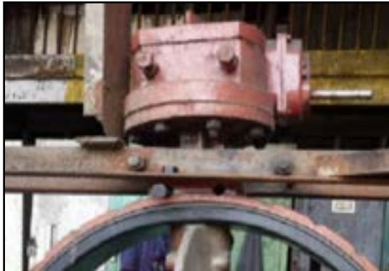
Seized butterfly volute due to gearbox failure.
