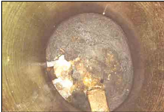
Hardened grease was causing pump burnout.
