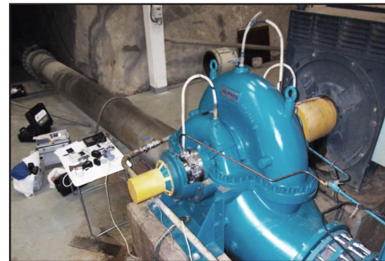
Reinstalled pump undergoing efficiency measurements
