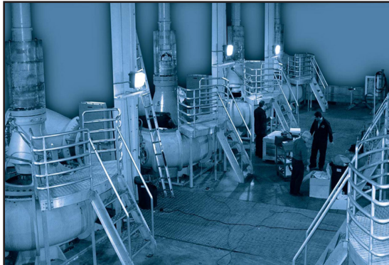
Large influent pump station.
