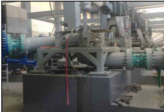
Dirt around the pump shows failure of original OEM dual seal.
