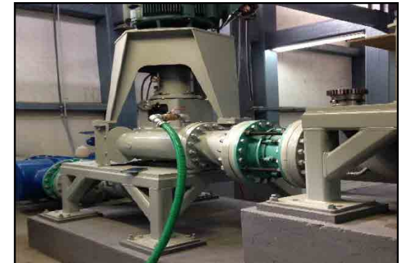
Pump and leak-free area with 442 installed.
