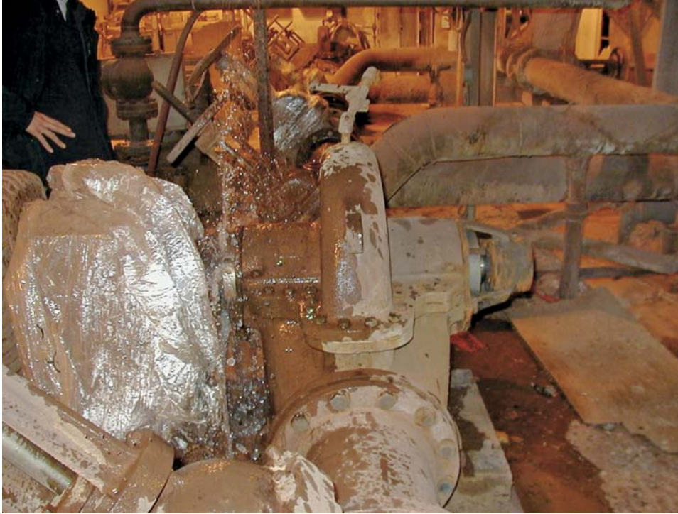
Past the time to fix the leak
