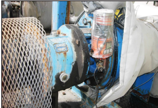
Greased SpiralTrac and packing on recycled ash water pump.
