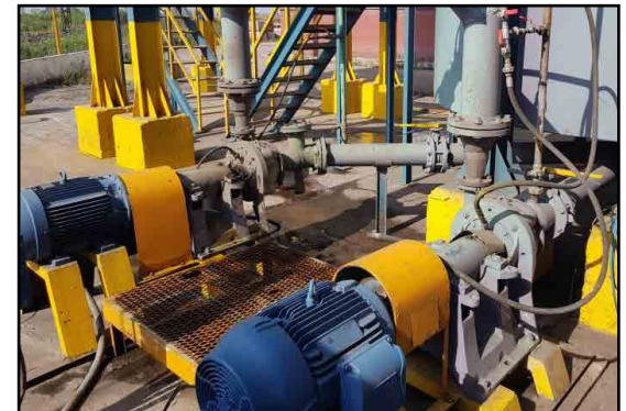
Pumps where packing was installed.
