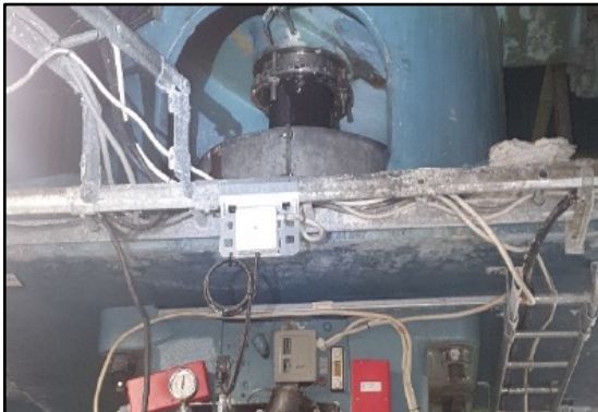
Oxygen Reactor requiring longer MTBR.
