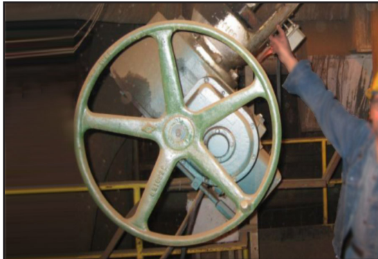
Steam isolation valve.
