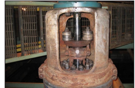
Critical plant valves have extended equipment life.
